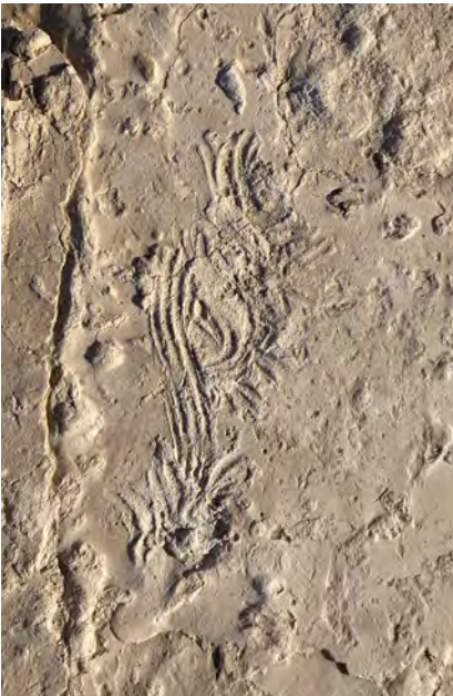
An exposure of the gypsum concrete foundations of the Long Temple where ancient setting ridges for talatat are visible along with swirling finger marks of an ancient concrete spreader
